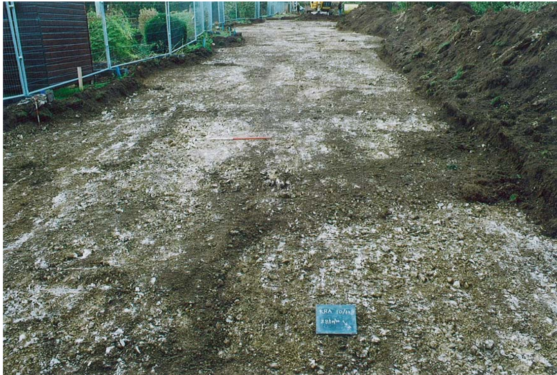
Plate 1. Stipping of initial road corridor of site adjacent to south eastern boundary, looking south west.
